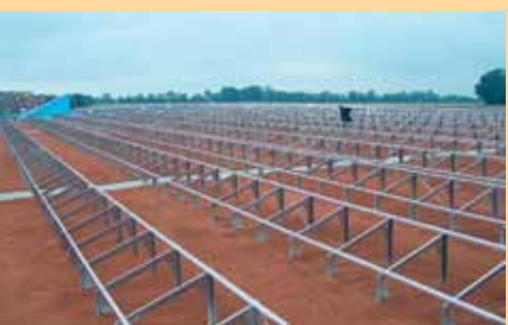
The Solar Base® plates are covered with system substrate as per the required load.
