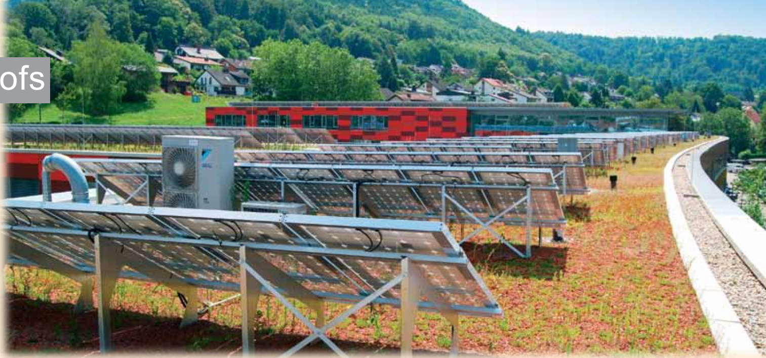
Photovoltaic system on a school building in Neckargmünd, Germany
