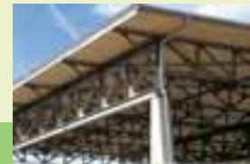
Low load bearing capacity
