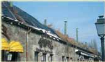
This photo shows the "Prussian Casemats" in Saarlouis before the refurbishment in March 2003. Tarps barely protect the building against penetrating precipitation.
