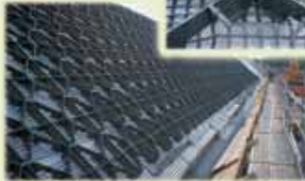
The roof's 45° slope is covered by stable high-tensile plastic nets. The Georaster elements are attached to the nets by stable cable binders.
