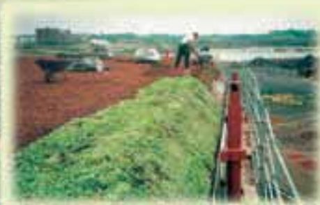
polymer roof covering, the green roof system has been installed. Supporting the concept of recycling, system substrate and drainage elements were made of recycled materials. A special challenge was the covering of the roof's perimeters with a 45° slope. The base, 120 mm eave profiles, manufactured of stainless steel, were built in for the edging.
