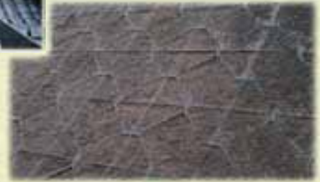
The special substrate had to be infilled, in a moist condition, and to avoid hollow space it had to be compressed, therefore enabling the installation of the pre-cultivated turf.
