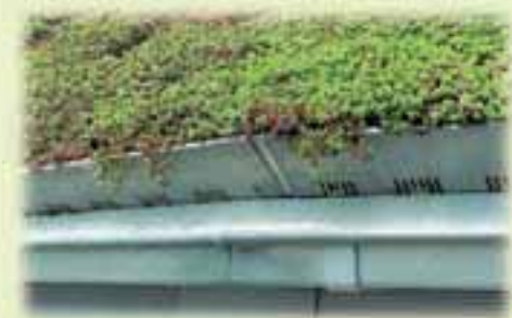
Floratec FS 75 elements and ca. 80 mm of System Substrate “Rockery Type Plants”, serve as a base for the installed Sedum vegetation mats.
