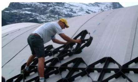
The Georaster® elements are installed from the bottom up. In the background, the Eiger north face.
